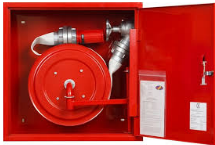
Figure 5.9: Fire hose reel
