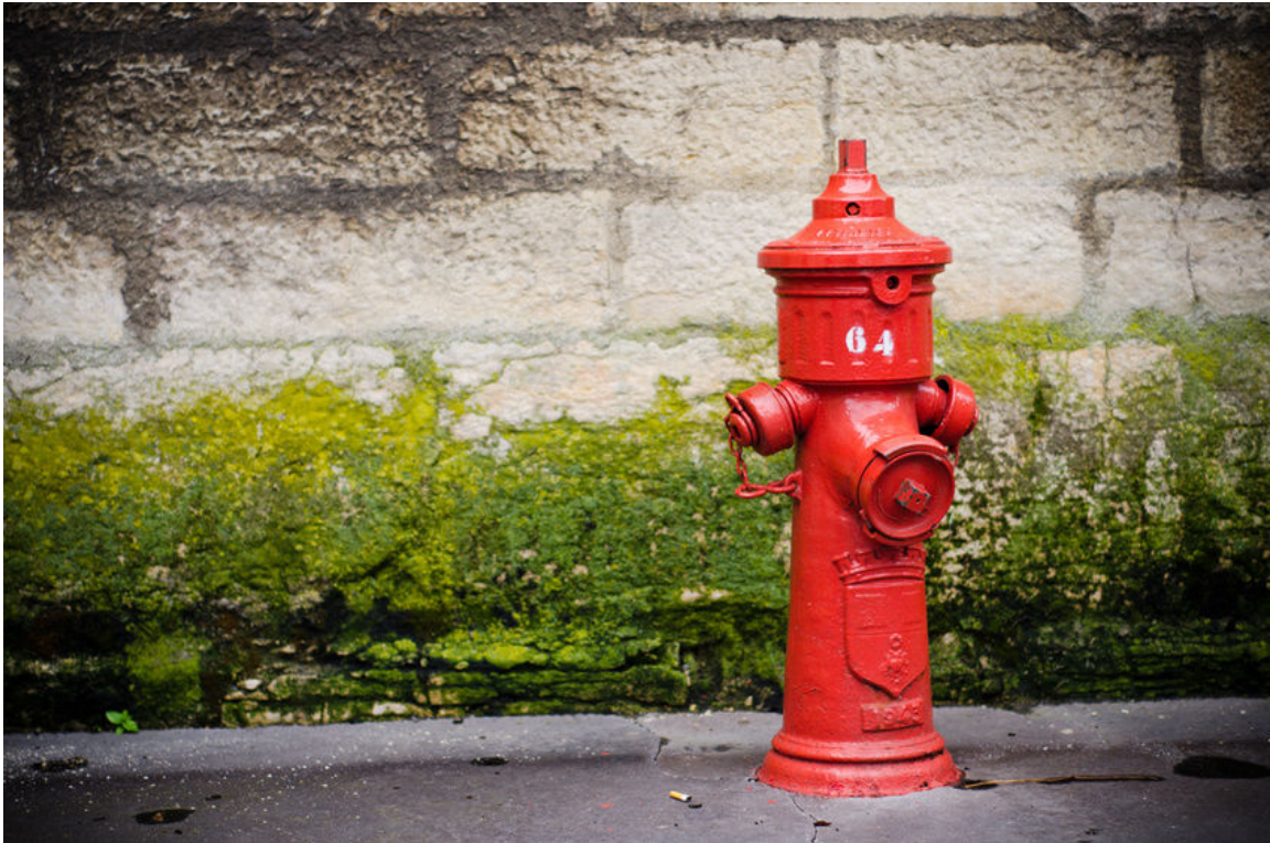
Figure 5.10: Fire hydrate system
