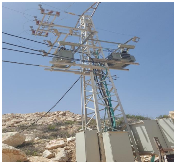
Figure2.5: high voltage towers
