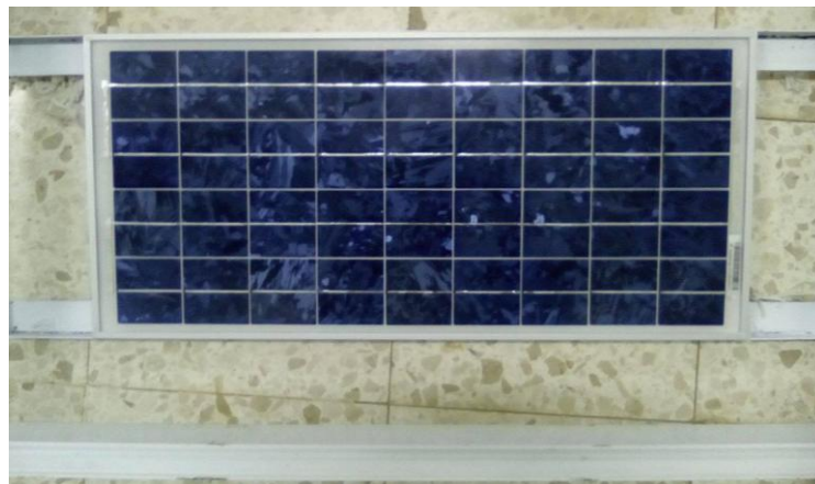
Figure 4-7: 20 watt solar panel used in project
