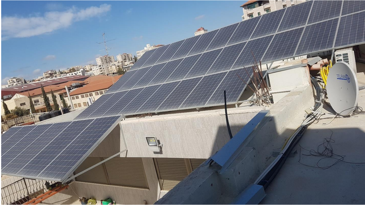
Figure B-5: 30 KW PV station.
