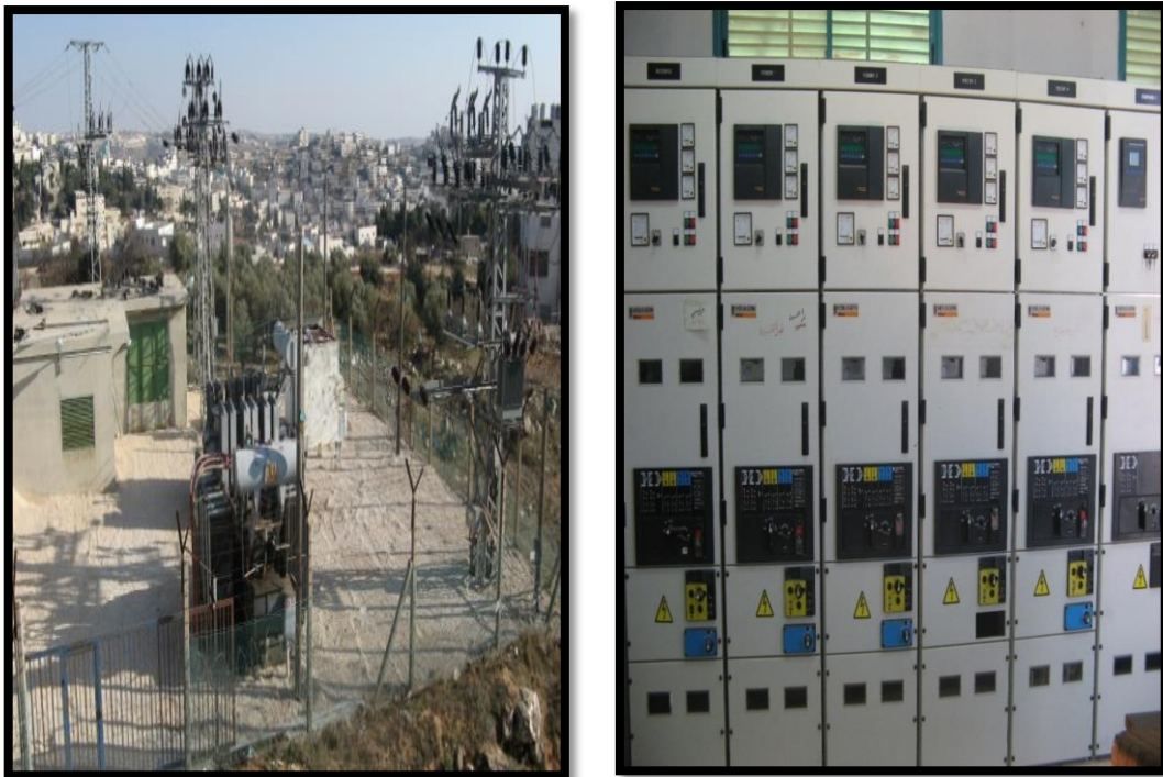
Figure (2.10) :( a) Power Transformer (b) Switchgear in Alras (S/S)
