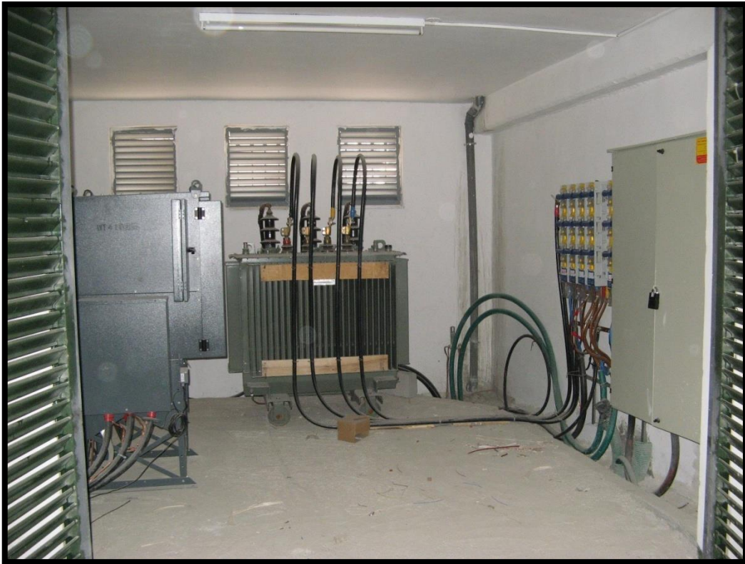
Figure (2.21): Distribution Stations in Hebron Electricity
