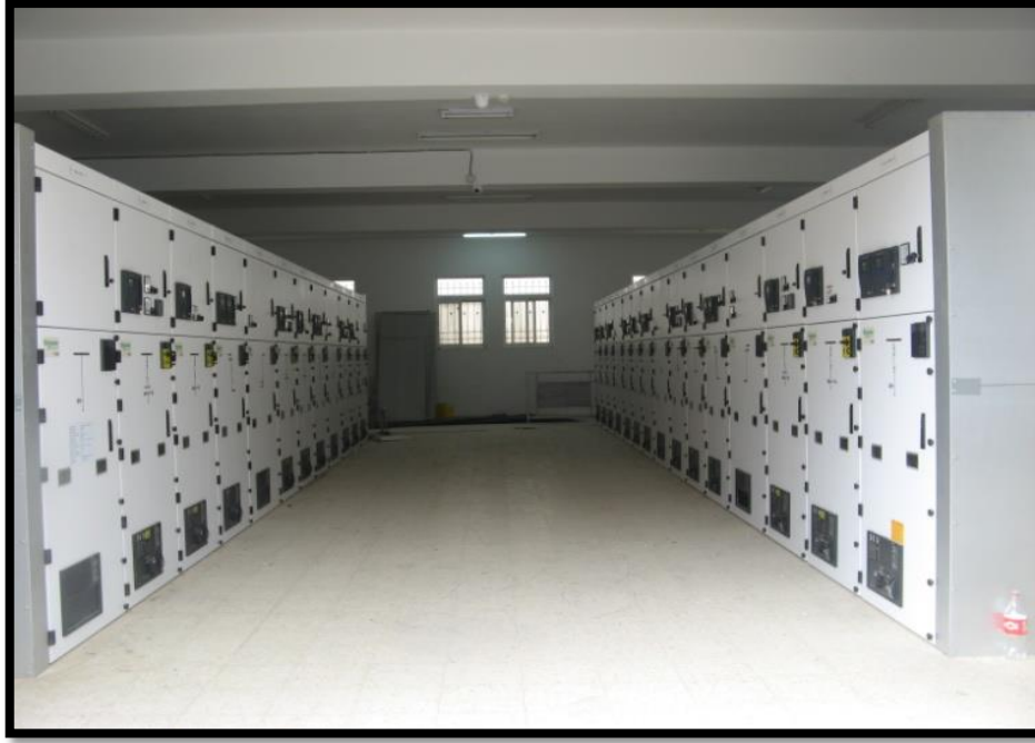
Figure (2.4): Main Power Control (MPC) Substation
