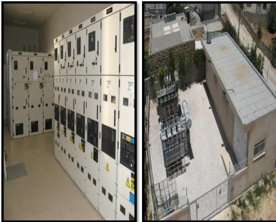
Figure (2.14):(a) Switchgear in Alhusein(b): Power Transformer in Alhusein (S/S) (S/S)
