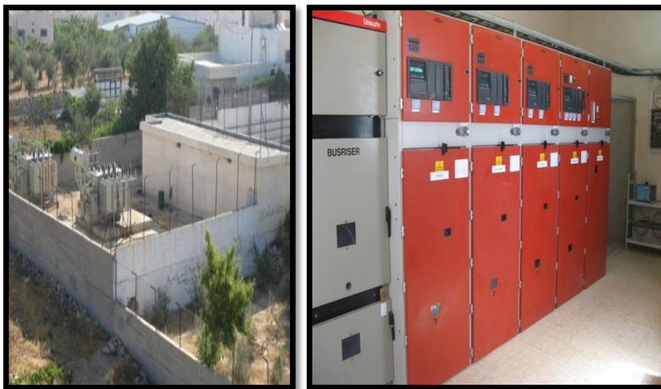
Figure (2.18):(a) Power Transformer in (b) Switchgear in Alharaq S/S
