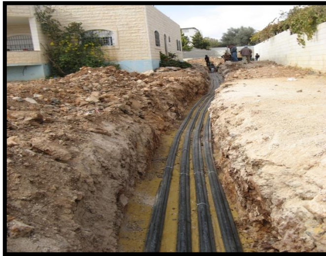
Figure (2.19): Underground Cable
