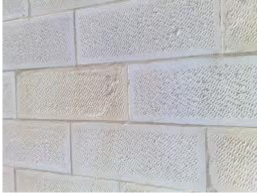
Figure(1.3): Distance between the stones not equals.
