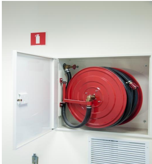
Figure 5.2: Fire hose reel
