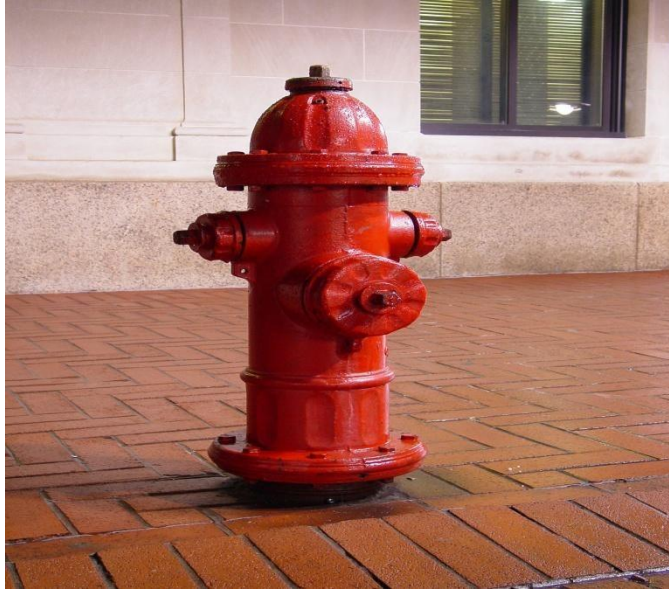
Figure 5.3: Fire hydrate system
