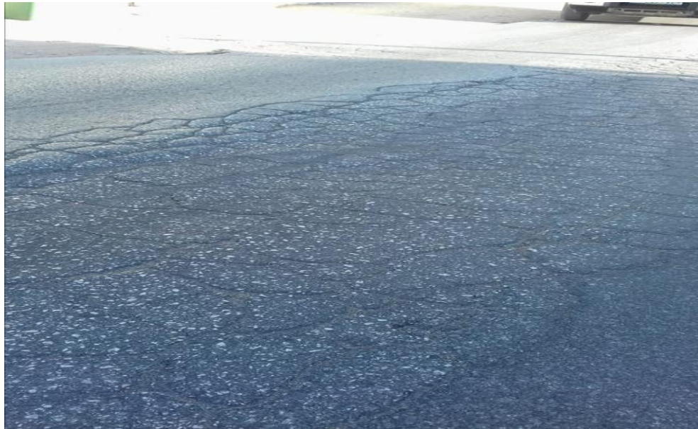
Photo (2): Asphalt Crack Event
