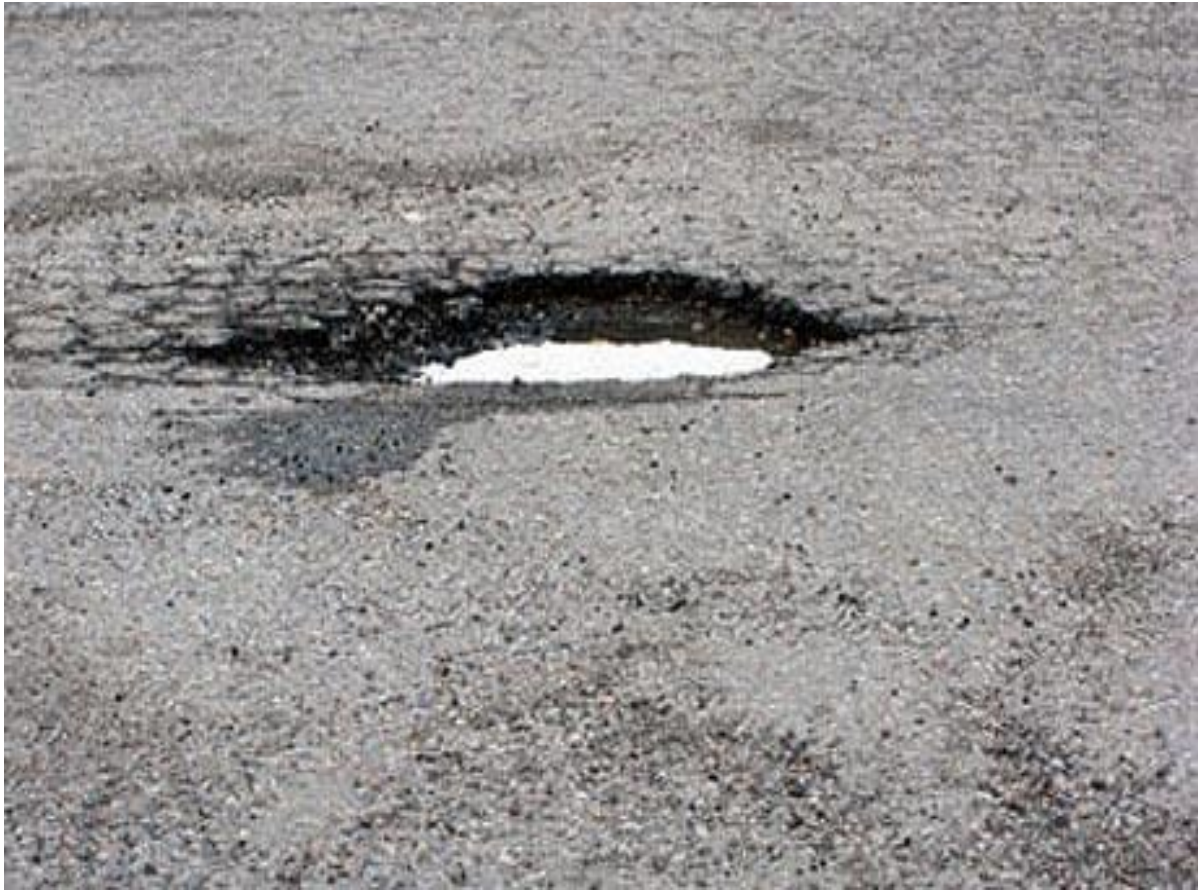
Photo (4): Hole Event in the Middle of Street
