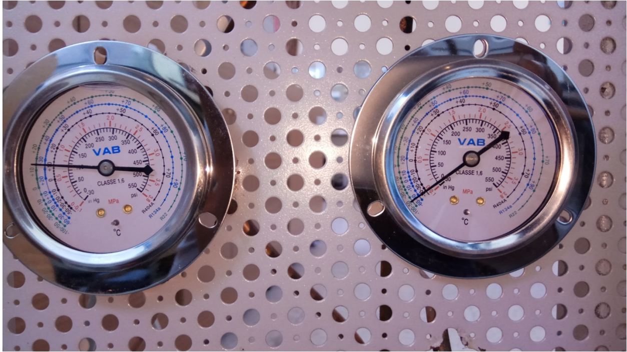
Figure 5.4 show the low side pressure and the high side pressure when using the conventional ON/OFF controller.
