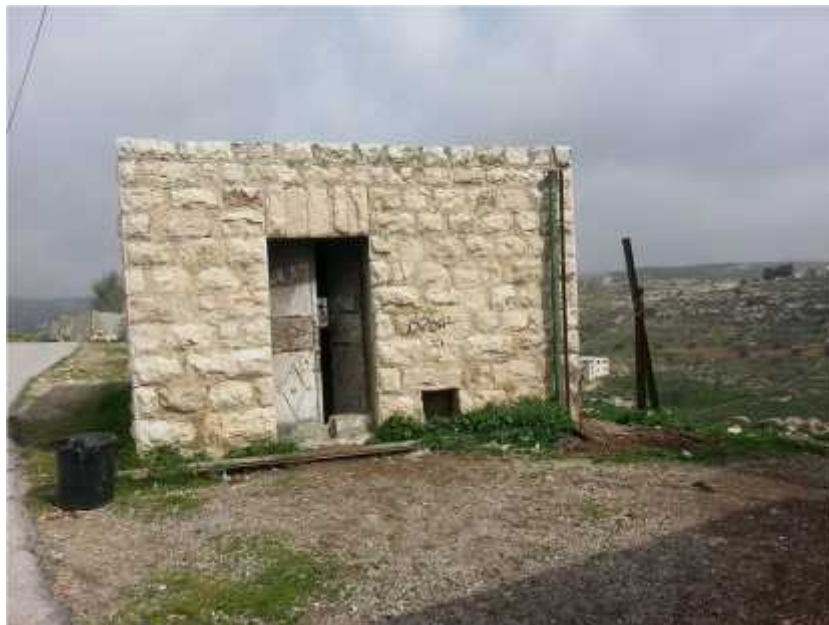
Figure 4.17 : building in poor condition.
