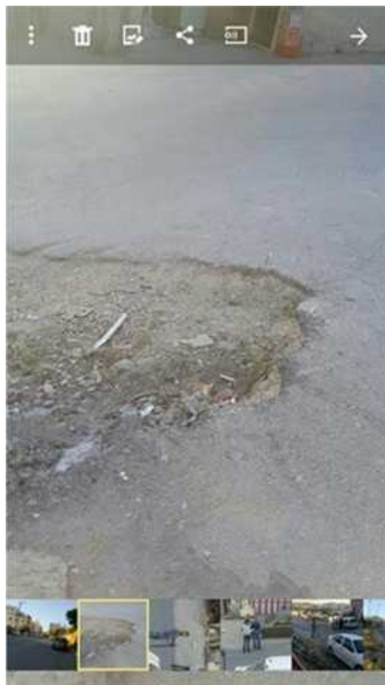
Photo 4: Hole Event in the Middle of Street
