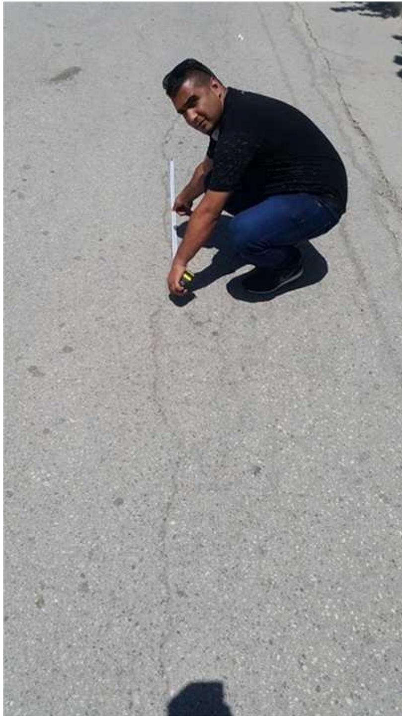
Photo 2: Asphalt Cracks Event
