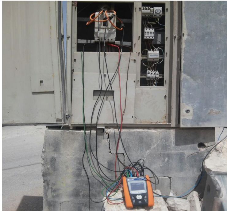
Figure 3. 7 Vega on transformer box.
