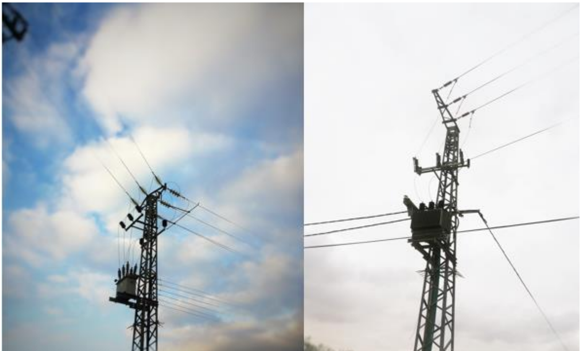
Figure 2. 4 High voltage towers.
