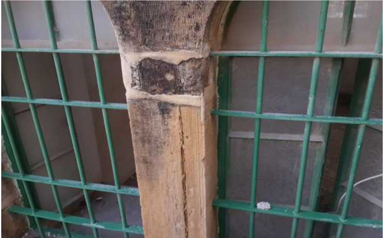
figure 7.5: the windows of the building needs renovation Source : by the researcher .
