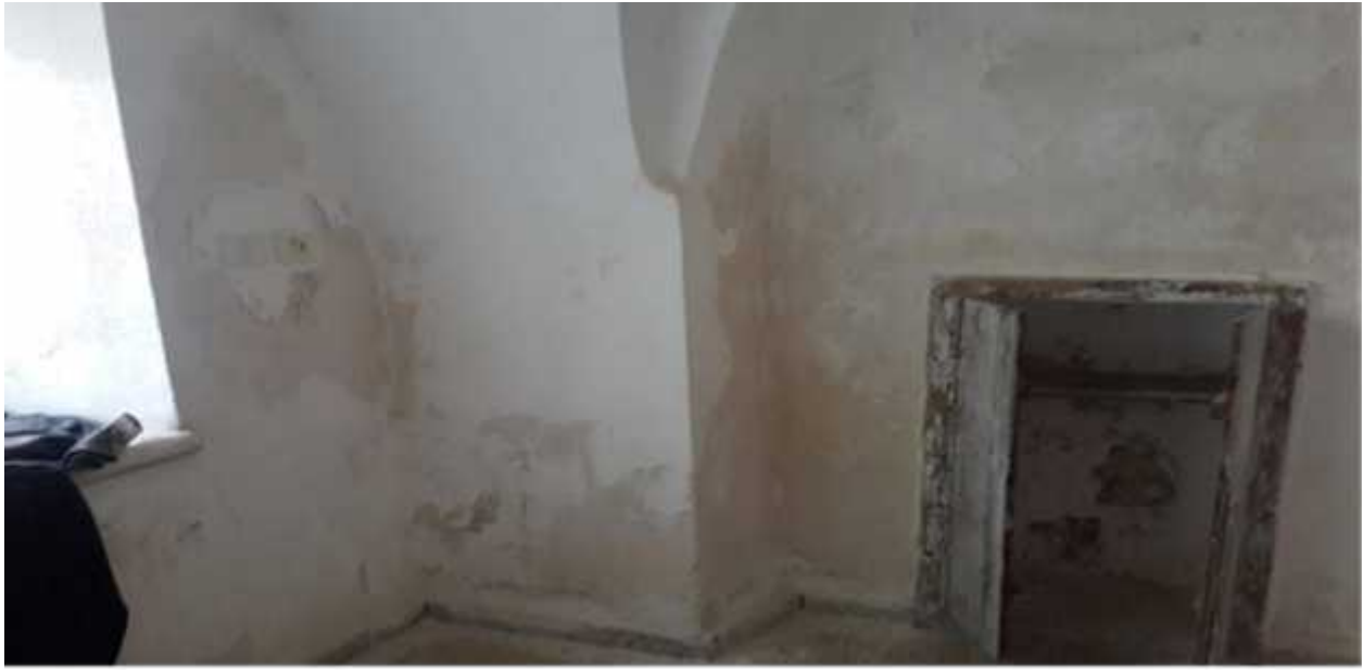
Figure 7.1: We will renovate the room by suitable kind of paints . Source : by the researcher .
