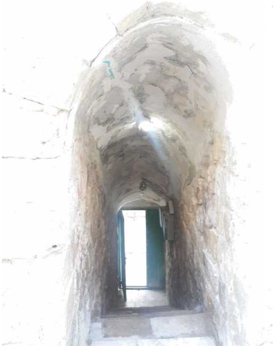
figure 7.5: the intrance of the building needs renovation Source : by the researcher .
