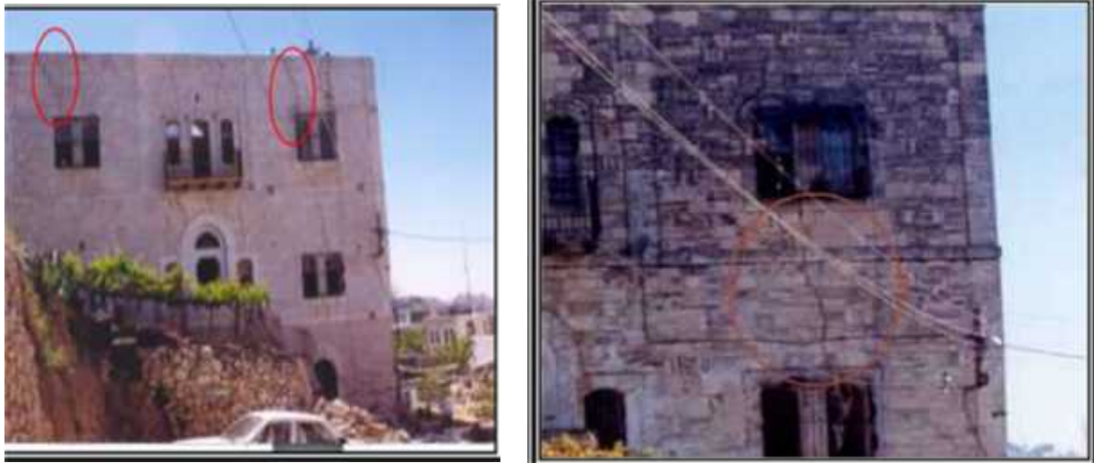
Figur 5 : shows the elevations before the renovation and the cracks appear clear in it .
