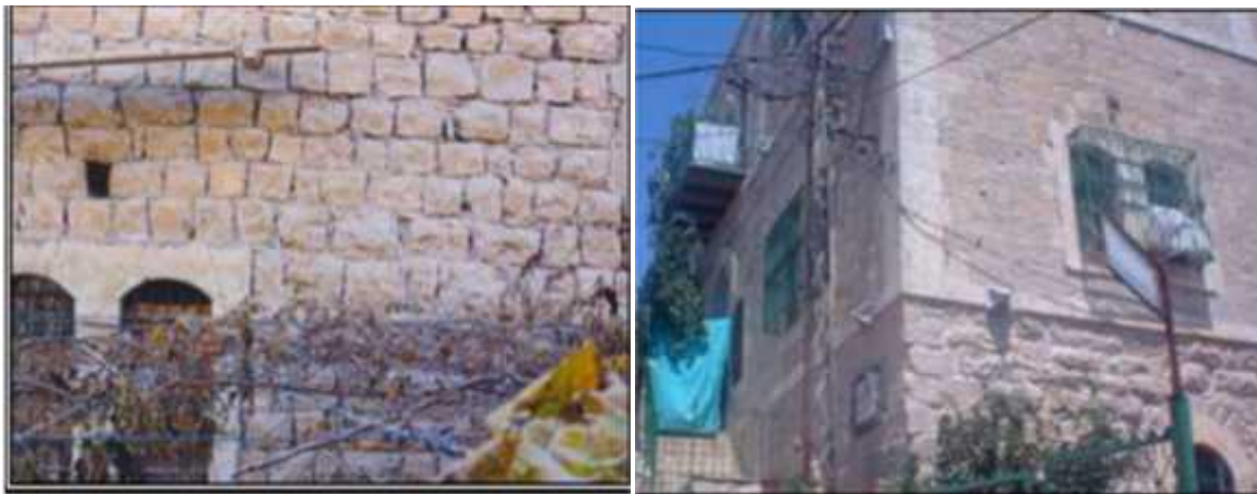
Figur 9 : the picture on the left shows the building before renovation and the picture on the right shows it after renovation .
