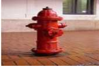
Figure (4.7) Fire hydrant
