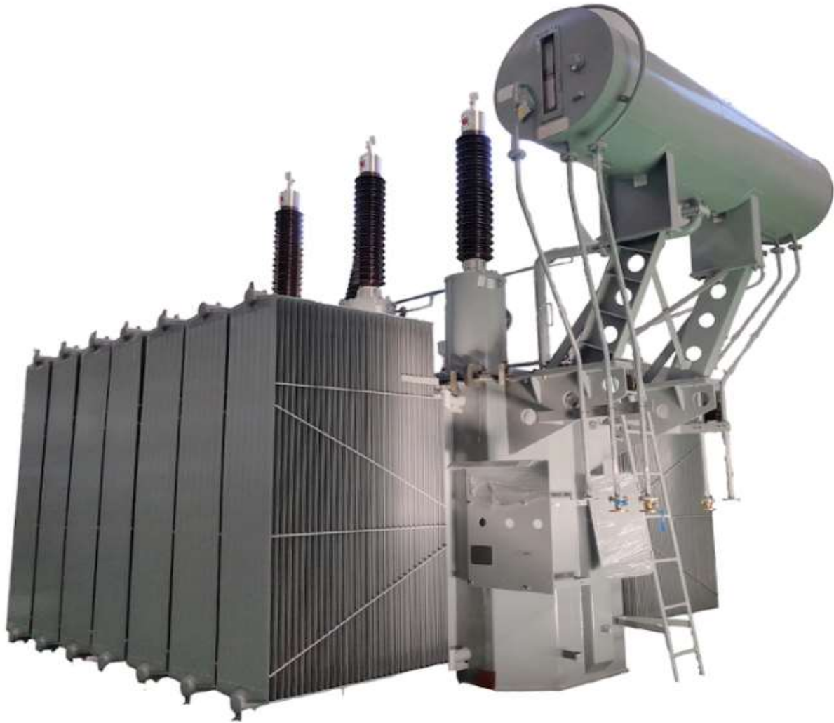
Figure 2.4: 161/36 KV 50 MVA power transformer
