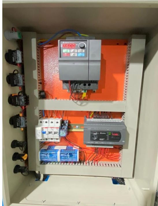
Figure (5.3): Machine Control Panel From Inside
