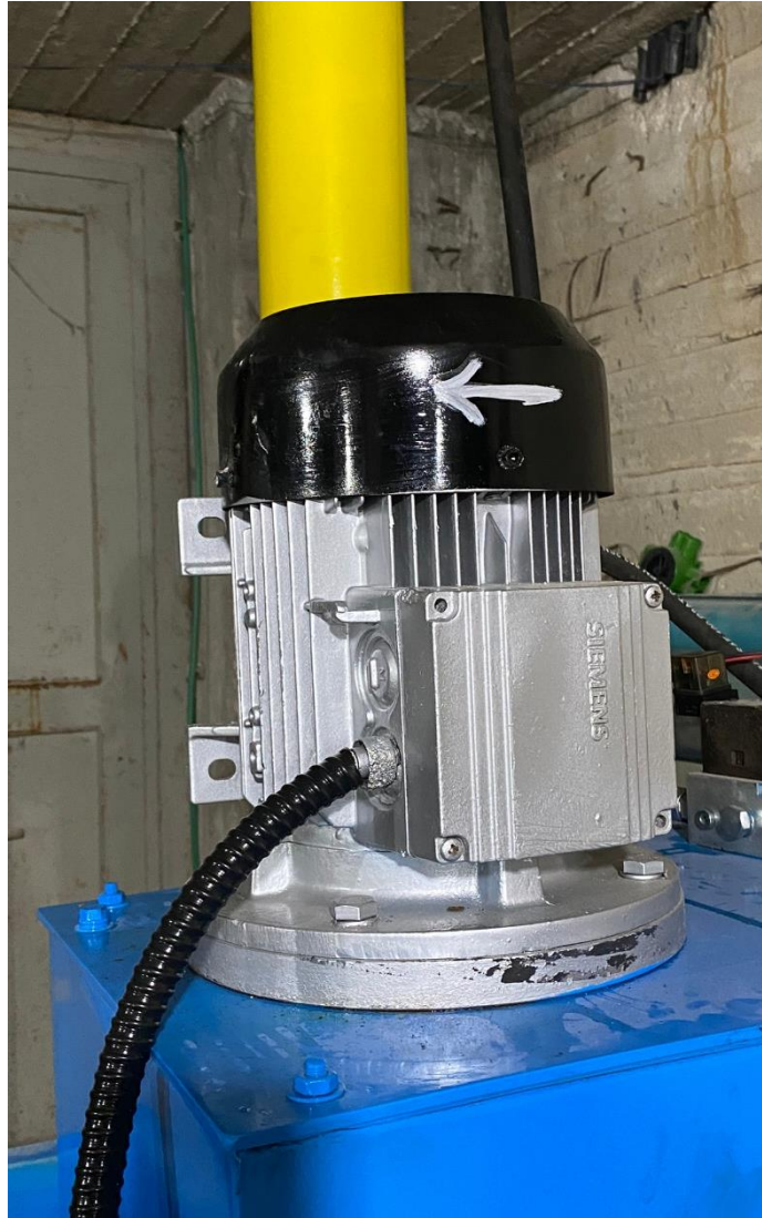
Figure (5.5): Motor for pump unit
