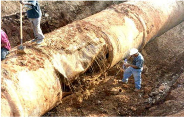
Fig. 2 Transient-caused failure, Super-aqueduct of Puerto Rico
