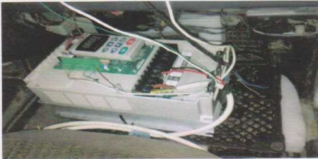
Figure 7:13 delta variable frequency converter type VFD-F 15 KW
