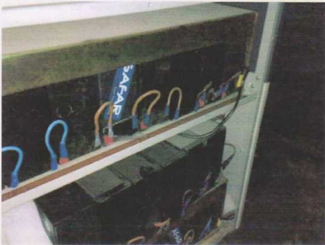
Figure 7.12: Lead acid batteries connected in series
