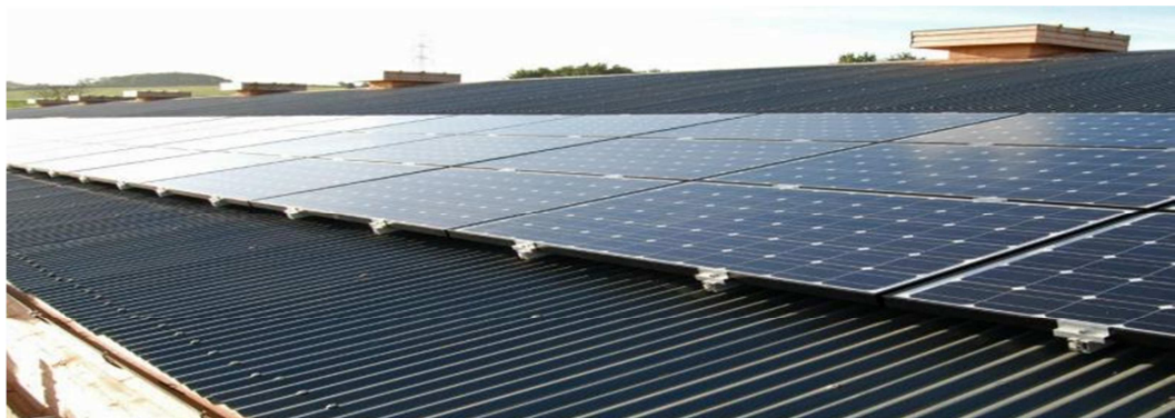
Figure (1.10) “PV system “
