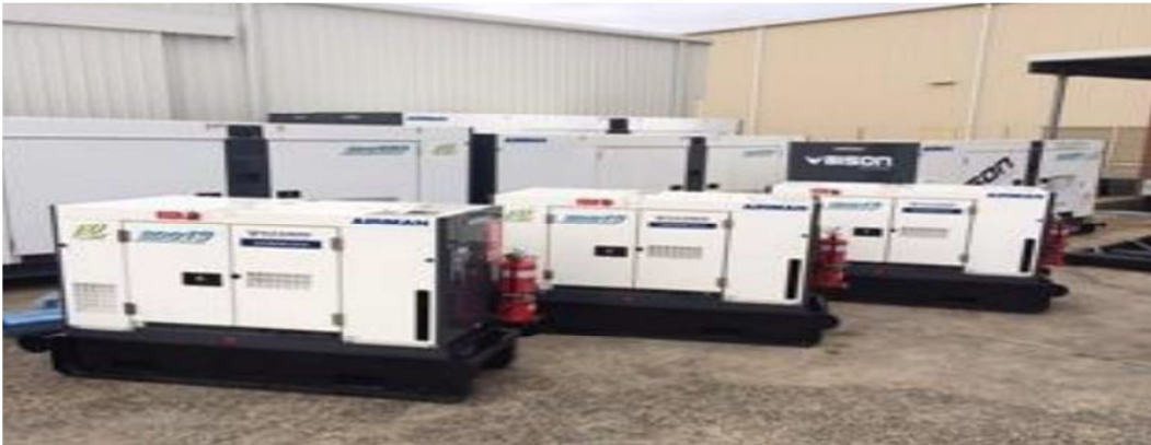
Figure (1.11) “Auxiliary generators stand-by”
