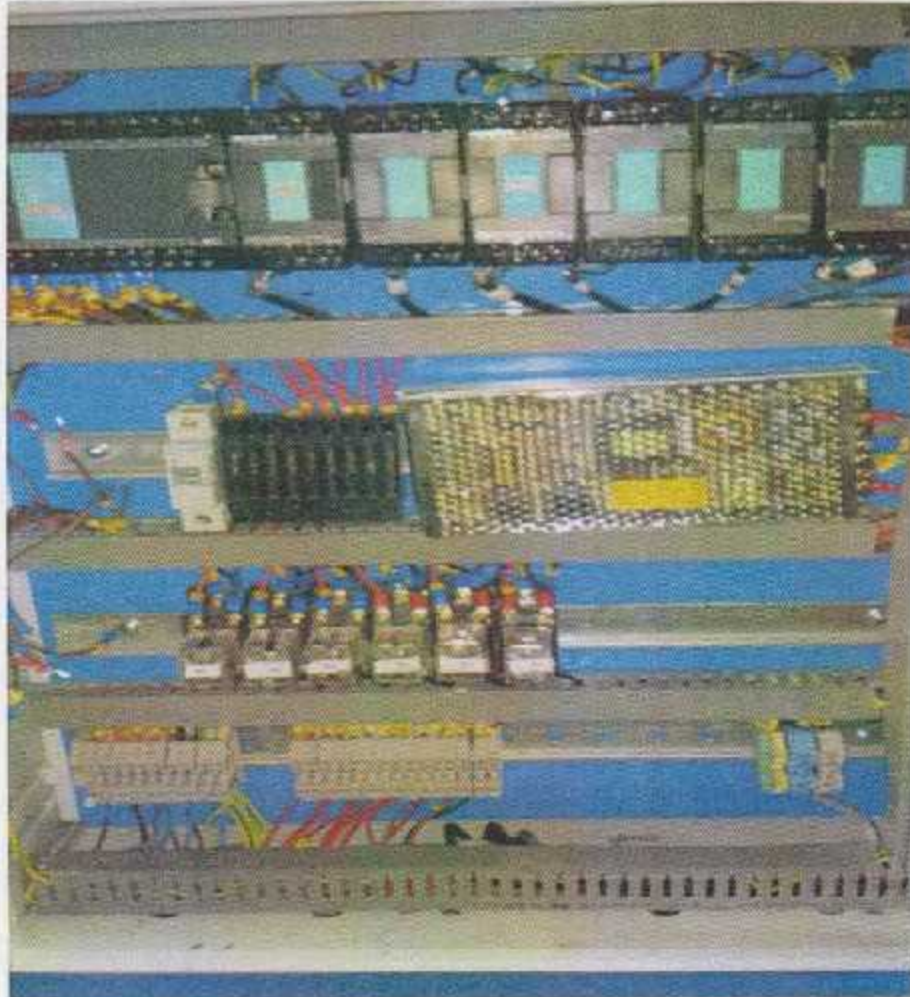
Figure (5.8): The Panel Electricity
