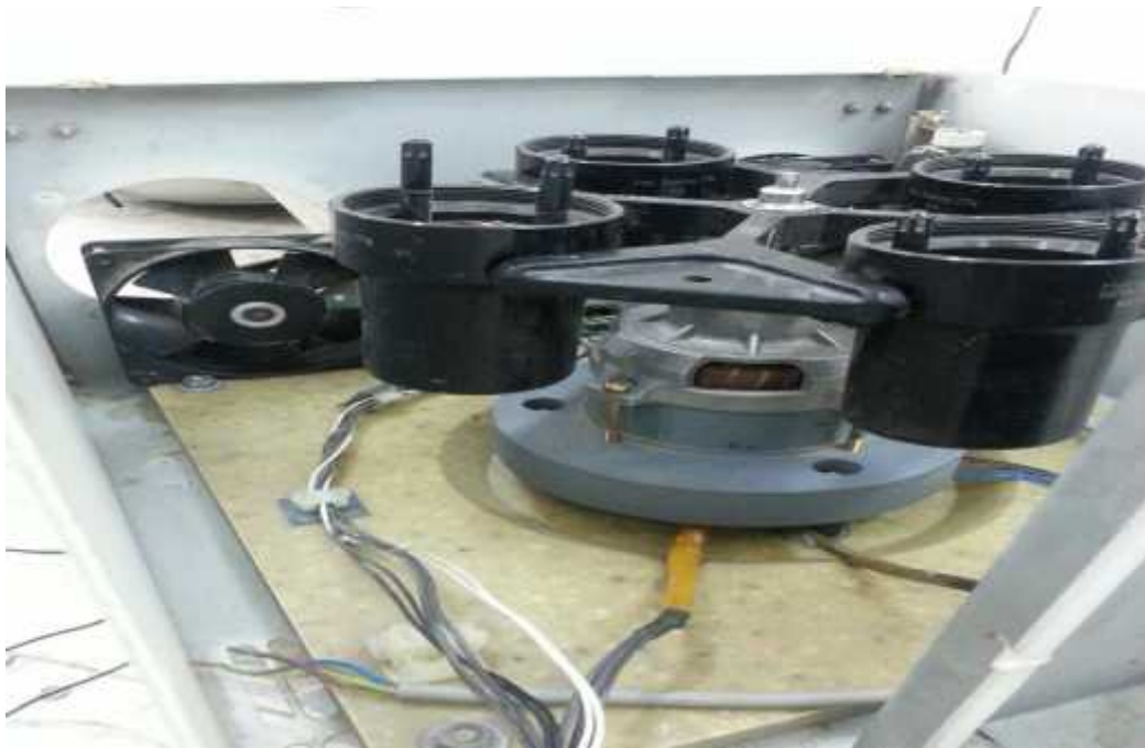
Figure (4.2): Three phase AC Motor
