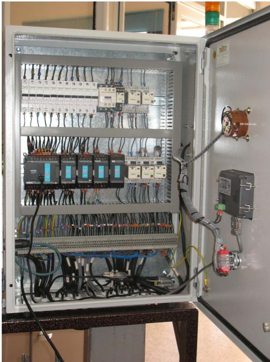
Figure (4.23): Electrical Board of the Machine
