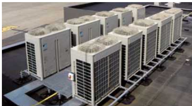
Figure (6.2) Outdoor unit
