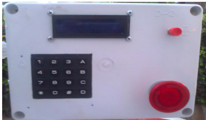
Figure (5.2): Control panel.
