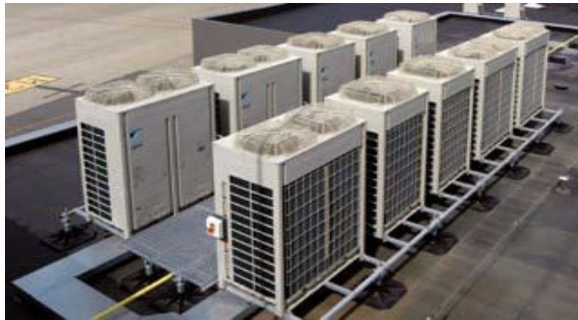
Figure (2.15) Outdoor unit
