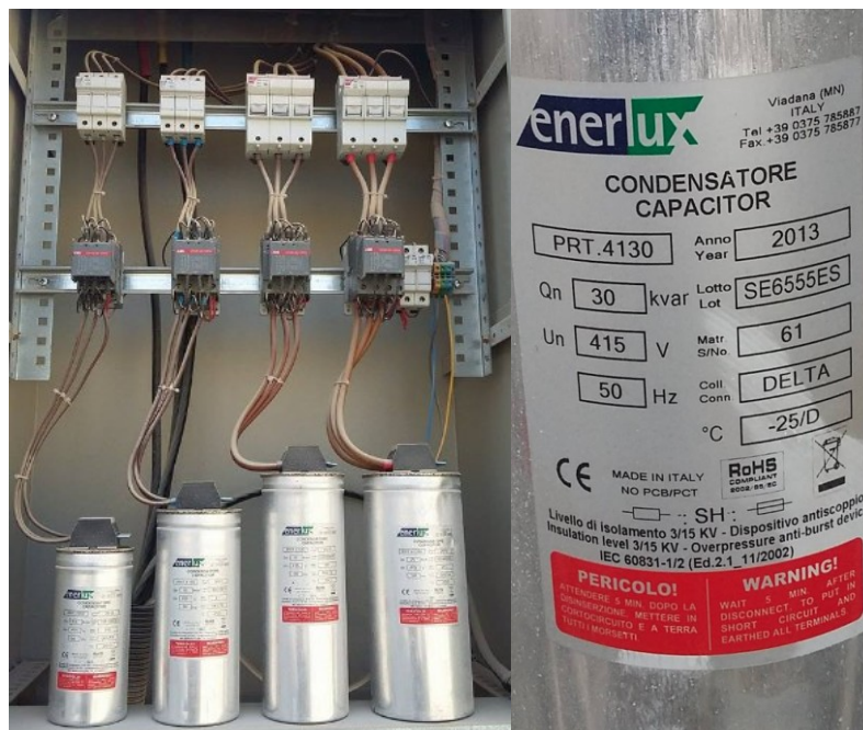
Fig. 2.10 Capacitor bank and plate name.
