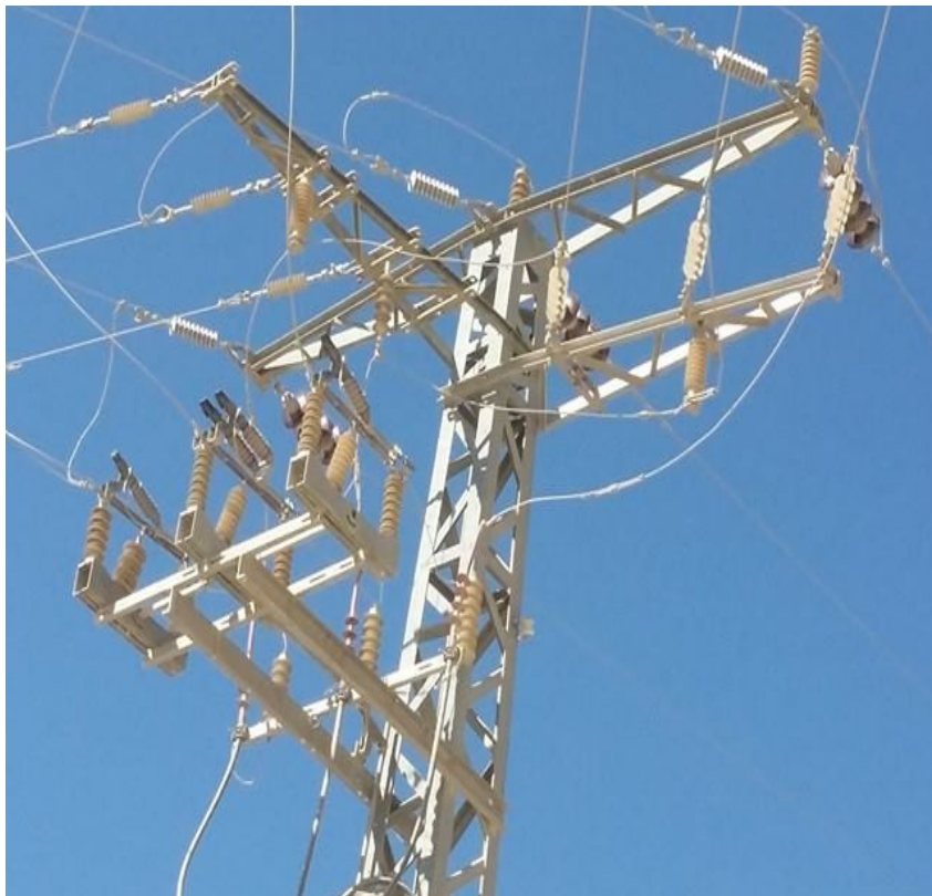
Fig 5.4: Isolator is not clean and dirty.
