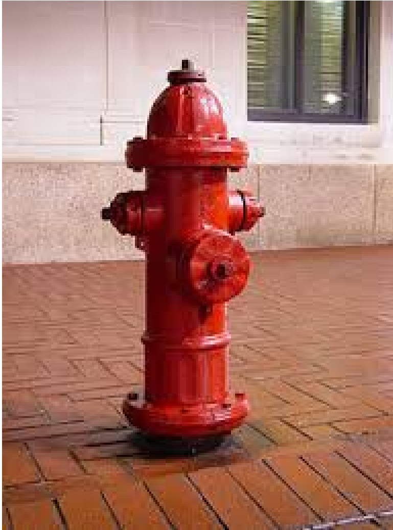
Figure 5.3: Fire hydrate system
