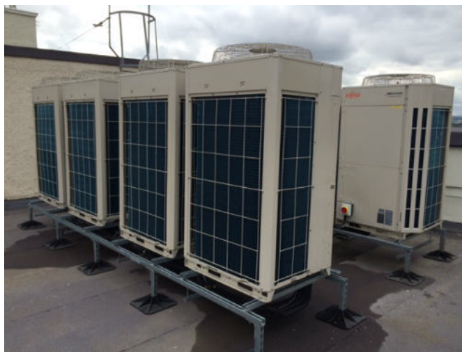
Figure 3.5: Out door units
