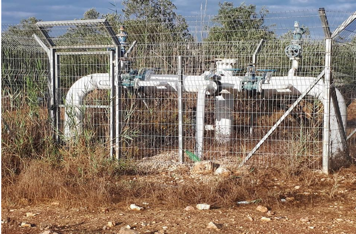
Figure 2.4 :The bukaa- tank( Main pipe)
