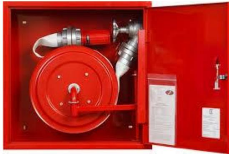
Figure 11: Fire hose reel
