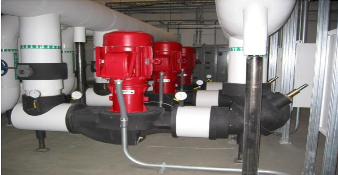
Figure 5.6: Inline fire pump
