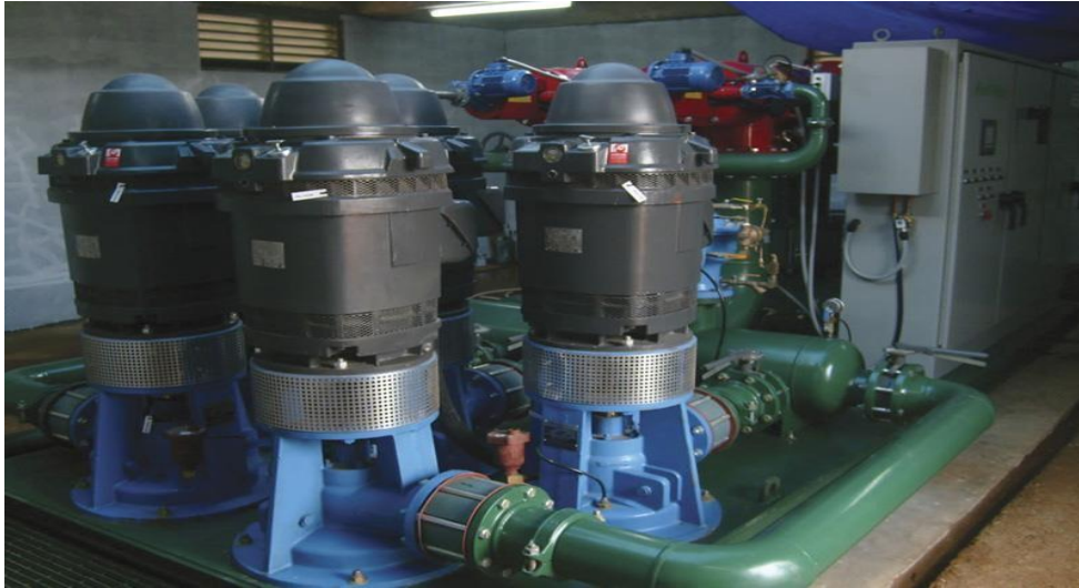
Figure 5.8: Vertical turbine pump
