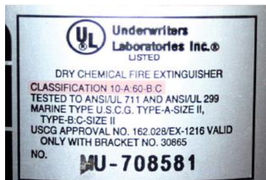
Figure (5.3) Extinguisher label
