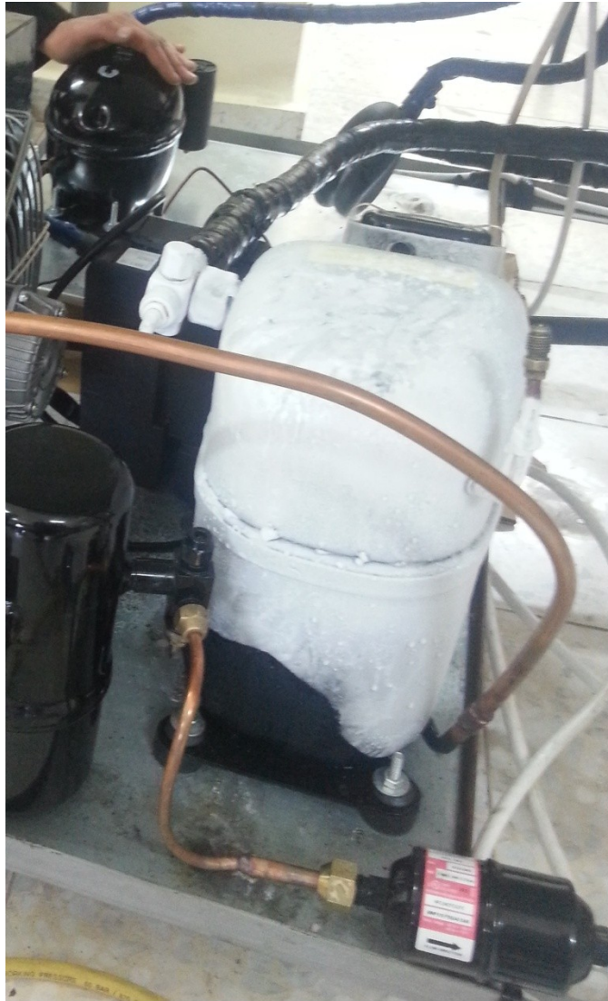
Figure 8.3 High Cycle Compressor
