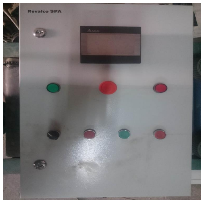
Figure 5.2: final control panel
